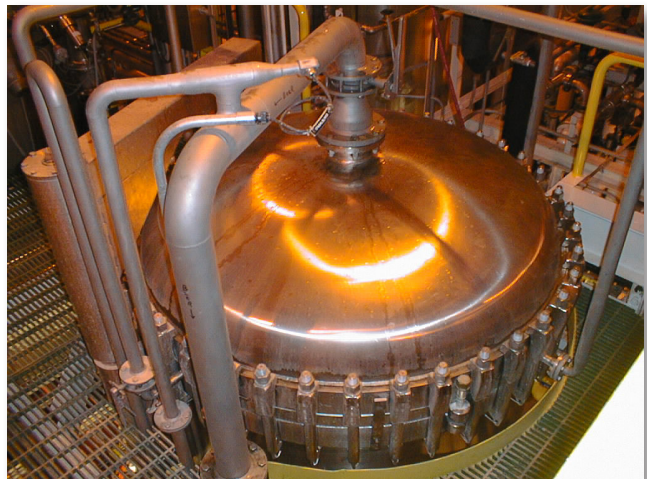
Process piping to brewing tank
