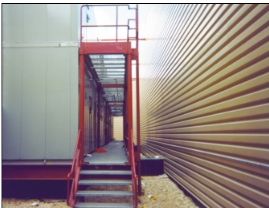
AHU Service Platforms
